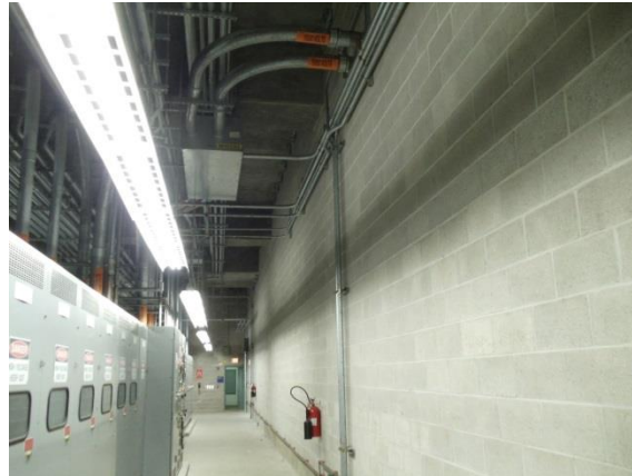
Vent Building 4– Detail of 15KV Electrical Conduit
